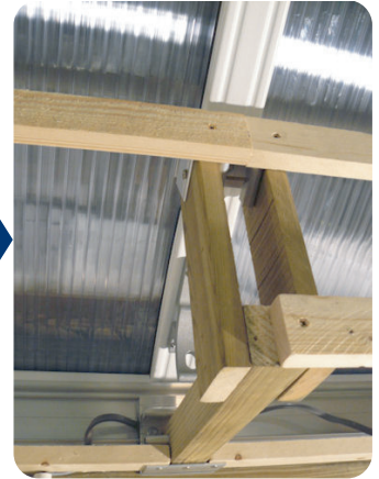
Complete the framework and ensure Tiewire can gain access to the bracket
