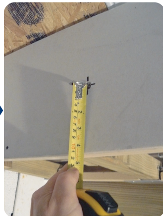
Attach the vertical plasterboard and transfer this size to form the 14mm dia. access hole
